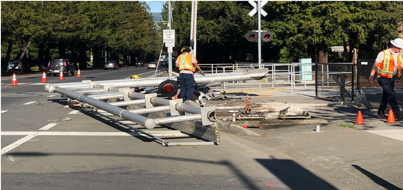
Signal knockdown at Rohnert Park Expressway
