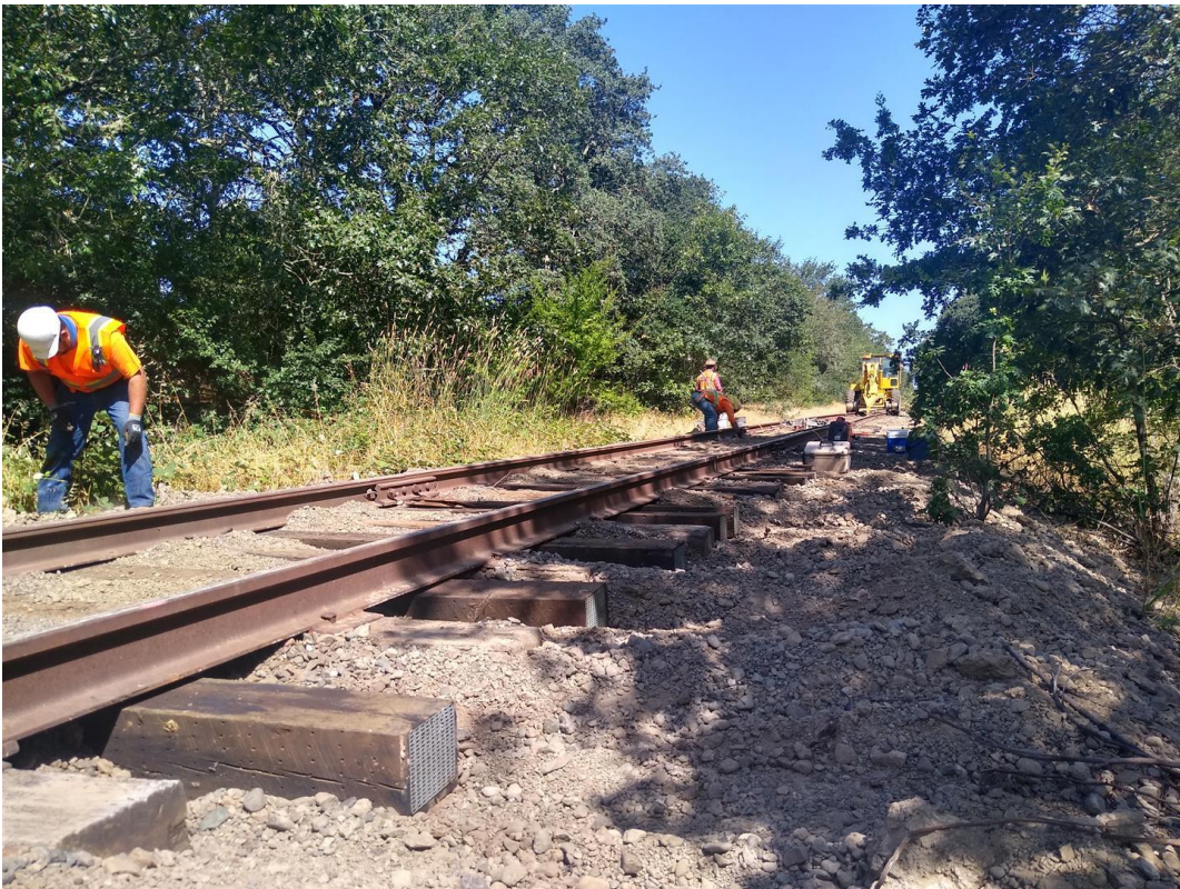
Replacing Ties at North End of the Project Between Windsor Road and Starr Road
